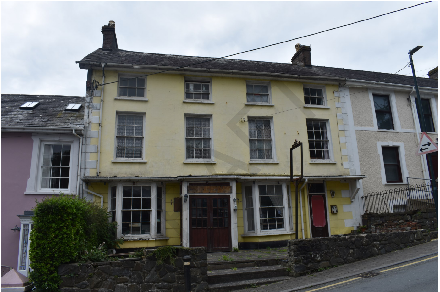
Fig. 12 The former Queen's Hotel is Grade II Listed but falling into disrepair
